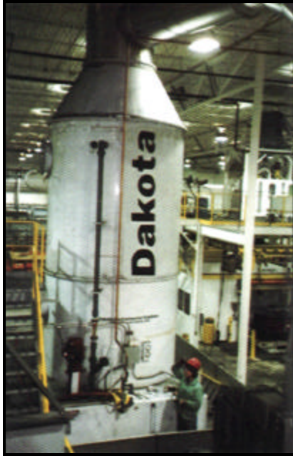
25,000 ACFM Dakota Scrubber™ removing dimethylethylamine (DMEA) emissions from phenolic urethane cold box process
