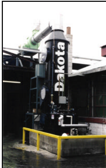
5,000 ACFM Dakota Scrubber™ removing triethylamine (TEA) emissions from phenolic urethane cold box process
